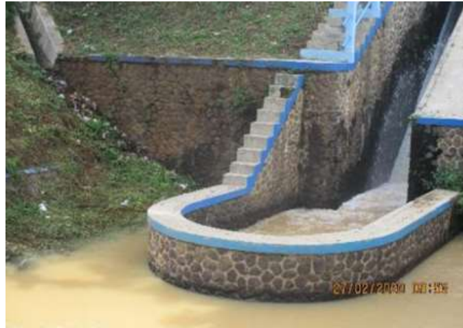
Figure 6. Condition of the Stilling Valve
