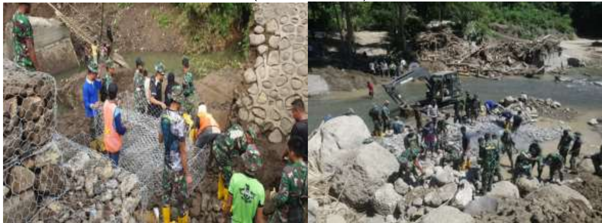
Figure 6. Civil Society Empowerment with the Indonesian Army in collaborative innovation of Ultra-Wide Acrow Panel bridge construction
