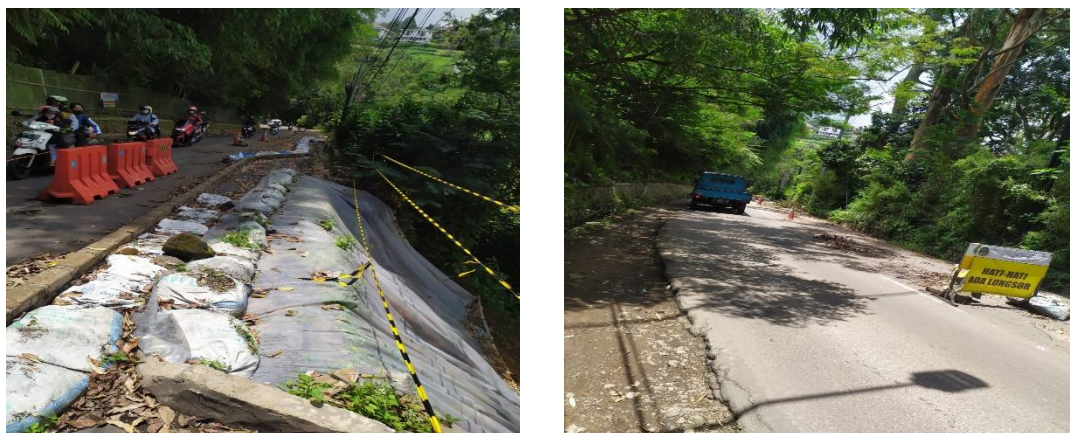
Figure 5. Condition Existing of Parongpong-Ngamprah Road
