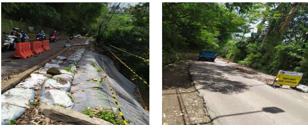
Figure 5. Condition Existing of Parongpong-Ngamprah Road
