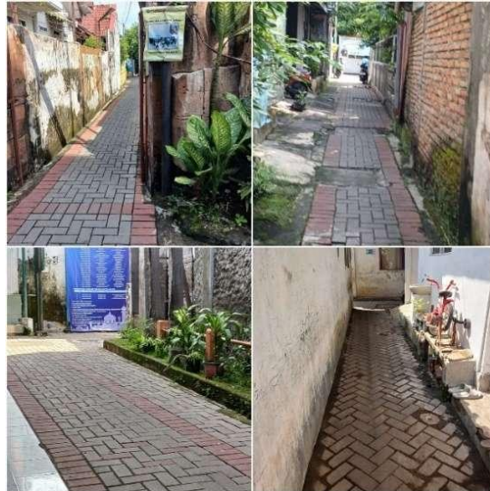
Figure 7: Road Conditions In Cokrodiningratan Village
