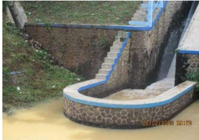
Figure 6. Condition of the Stilling Valve
